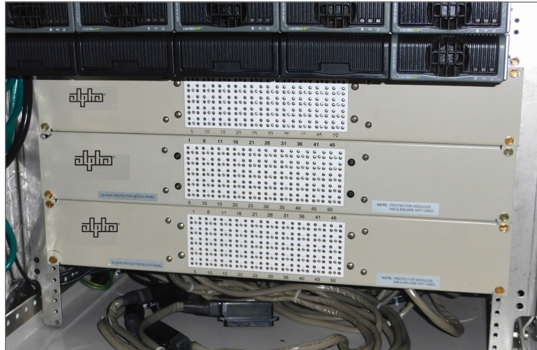
Figure 5: High voltage 50-pair protector panels
