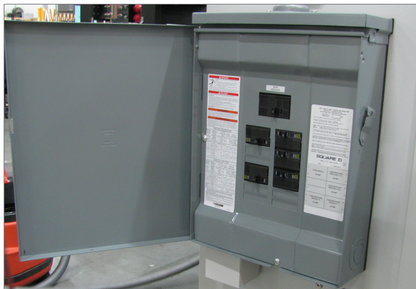
Figure 6: External AC loadcenter
