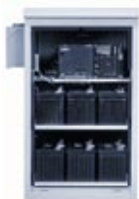
Single PN-3 1 Power Supply 2 Battery Strings
