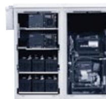
PN-4/CE-9X2 2 Power Supplies 3 Battery String AlphaGen™ Generator
