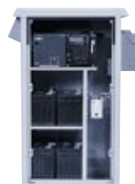
PN-SC-HS Sidecar 1 Power Supply 1 Battery String
