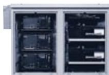
PN-6 3 Power Modules 2 48V Battery strings
