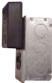
Fig. 5-10, LA-P+ Installed in BDO
