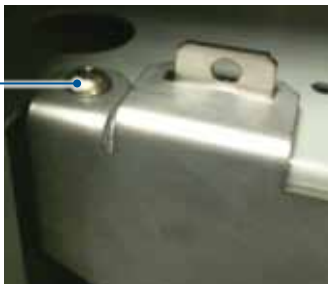
Battery bar attached with security screws and/or padlock
