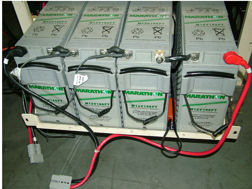
Fig. 1-11, Battery Storage Unit
