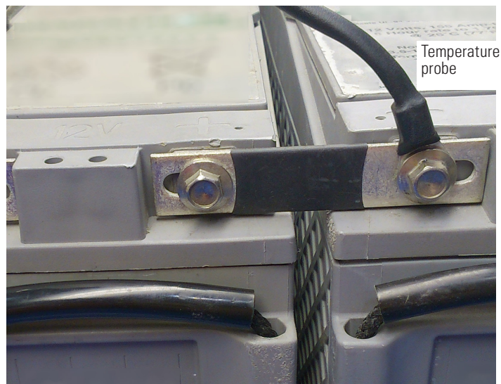
Figure 47: Battery temperature probes, battery bay
