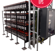
RACKS AND CABINETS
